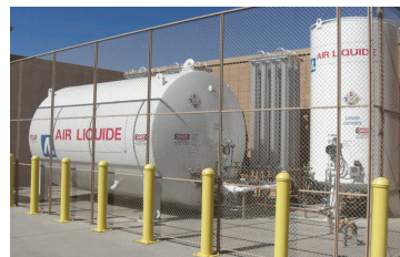
Bulk oxygen tanks currently monitored by iDATAL™
