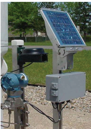
Installed DATAL™ by Air Liquide
