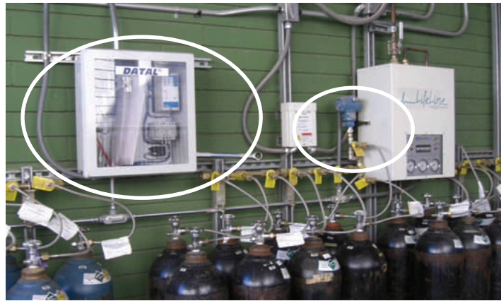
iDATAL™ panel (large circle) and transmitters (small circle) installed by Air Liquide on cylinder manifold
