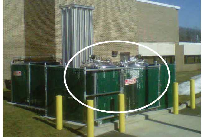
Air Liquide Oxygen VGLs installed at a customer’s hyperbaric treatment facility in the Northeast U.S.
